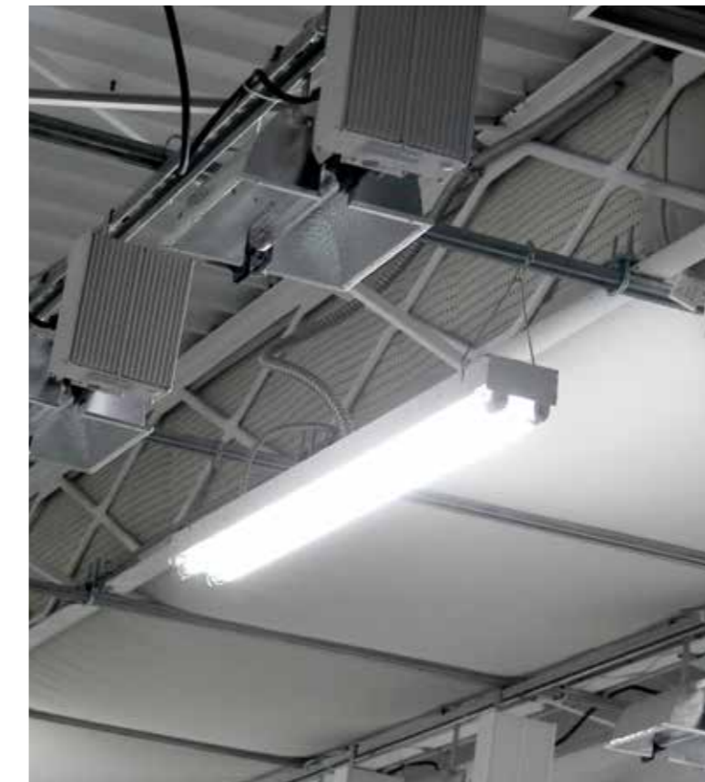
Rectangular duct between open web joist in an Ohio grow facility.
