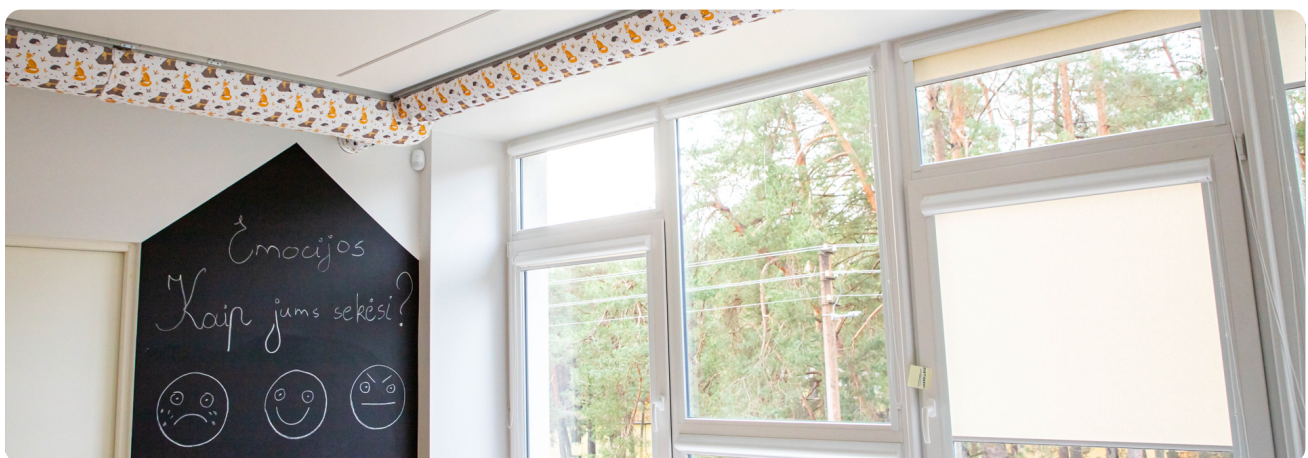
Machine-washable fabric ducting in an early-years classroom – the distribution system itself stays free of dust, allergens, and mold spores.
